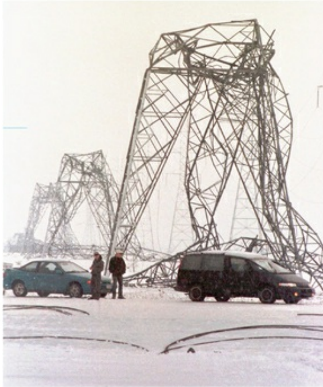
FIGURE 9.33 Transmission Towers Collapse Under Weight of Ice
