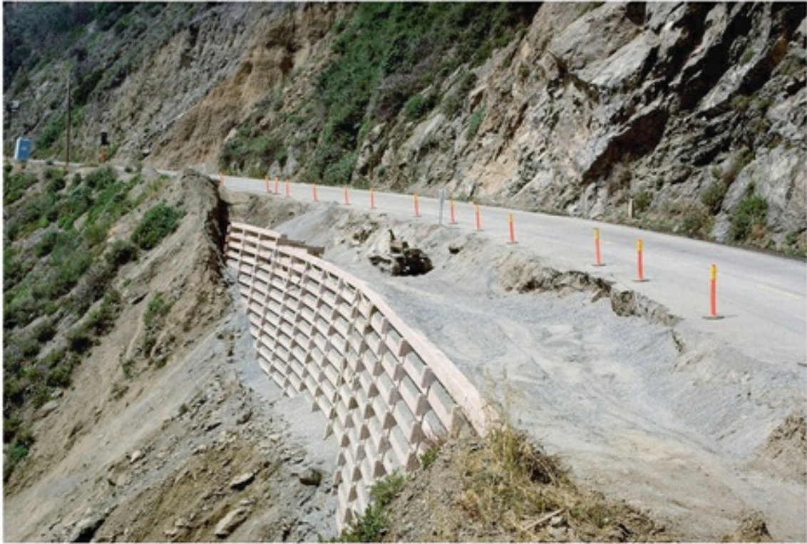
FIGURE 7.28 Retaining Wall This retaining wall of concrete cribbing was installed and then backfilled to help stabilize the roadcut. (Edward A. Keller)
