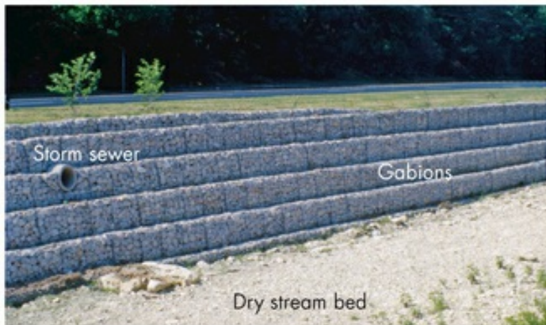
FIGURE 6.41 Gabions Stabilizing a Stream Bank These gabions along the bank of the dry streambed of Shoal Creek in Austin, Texas, are stacked baskets of metal chain-link fencing filled with rocks. They were installed to keep the stream from eroding nearby Lamar Boulevard. Their porous nature allows floodwaters and sediment to seep into the creek bank, thereby reducing the extent of flooding downstream and allowing plants to grow and partly cover the gabions. Nearly dry between rainfall events, the creek is also fed by storm sewers, such as the pipe in the left center. ( Robert H. Blodgett )
