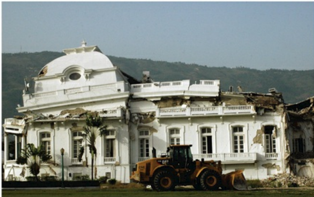
FIGURE 1.2 Collapsed Buildings in Haiti
