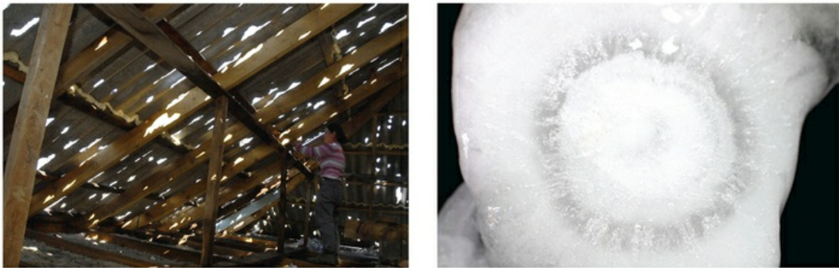
FIGURE 9.22 Hail Damage and Internal Structure
