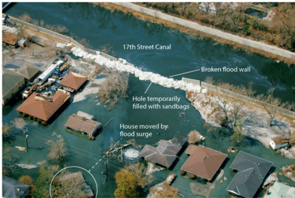
FIGURE 10.13 Aerial View of Temporary Repair of Breached Flood Wall and Levee on New Orleans's 17th Street Canal
